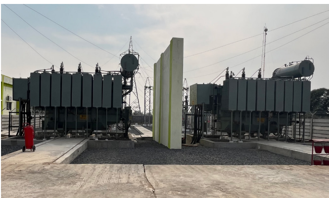
Fig.1. FR3 filled 2 nos. of 52.5/63MVA, 66/33KV power transformer placed at Sprng Ujjvala Energy solar plant in Banas kantha without NIPS system.
