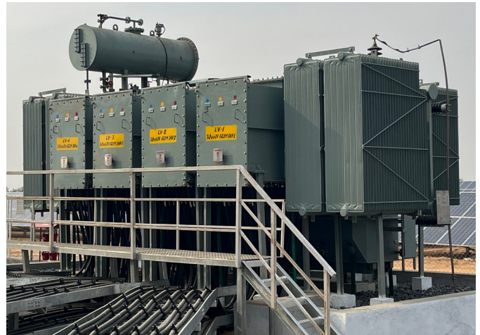
Fig.2. FR3 filled 10 nos. 12MVA ,33/0.63 KV IDT overloaded upto 13.125 MVA placed at Sprng Ujjvala Energy solar plant in Banas kantha.
