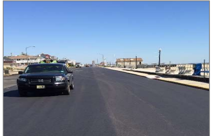
The left side of the road was paved with 45% RAP, 5% RAS and Cargill’s Anova™ Rejuvenator. The right side of the road was paved using only 20% RAP.
