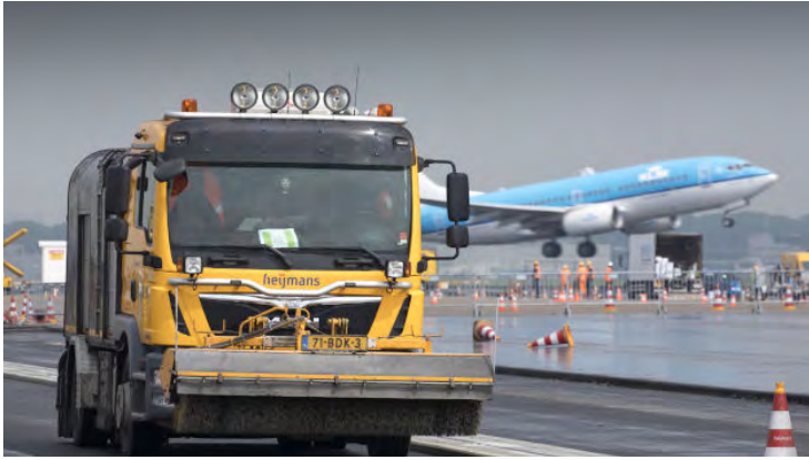
The products used needed to perform: the Polderbaan needed to be repaved with as little impact as possible on Schiphol's daily operations. © 2021 Heijmans
